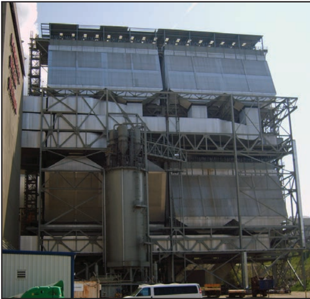
2 - 700 MW Coal Fired Units - ESP
