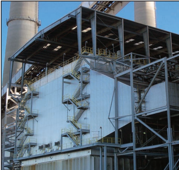
3 - 800 MW Coal Fired Units - ESP
